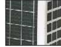
Evaporator during normal operation
