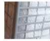
Evaporator covered with ice
